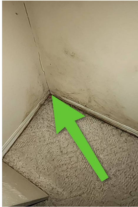
Swabbed closet wall intersection
